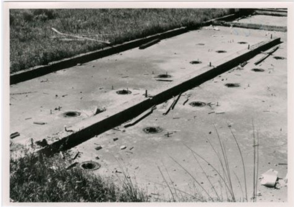
Toilet sewer holes in Tule Lake restroom and shower building. Photo taken c. 1983 by Harry Gamble and his team to lobby for Tule Lake to be designated a National Historic Landmark. Courtesy of the Frank Sato Collection, Densho.
